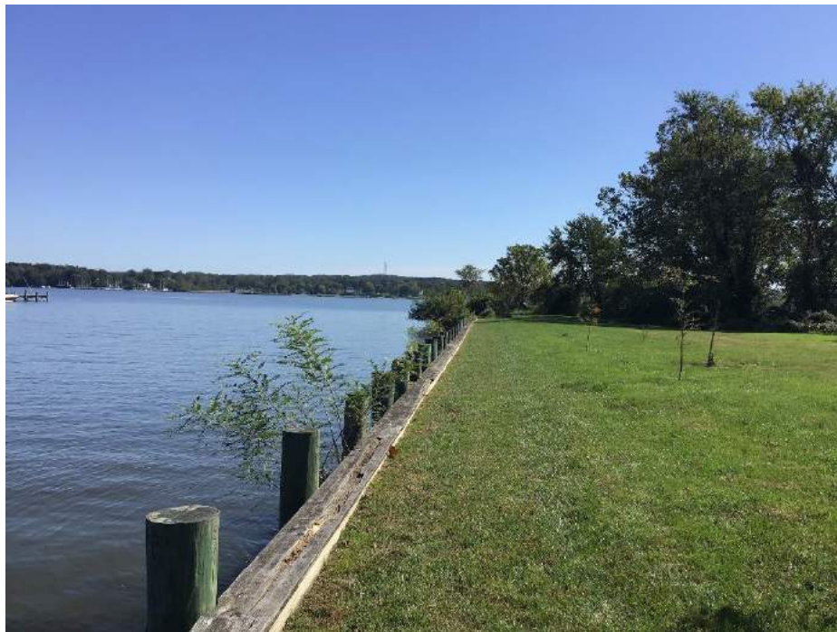
Photo 2: Existing bulkhead looking south towards the North East River and end of peninsula
