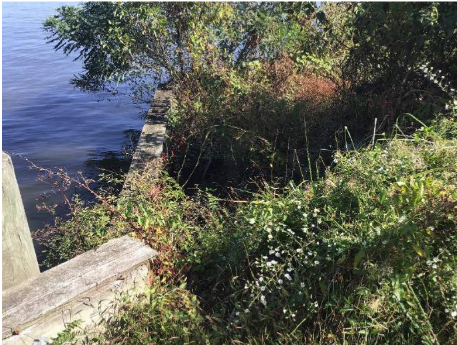
Photo 4: Erosion behind failing bulkhead
